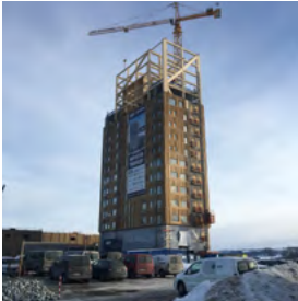
Stacked volumetric timber modules fit inside a mega-frame of prefabricated glulam trusses for this 14-storey apartment block in Bergen, Norway. The team cited a two-month shorter construction programme compared to conventional on-site methods. 75
